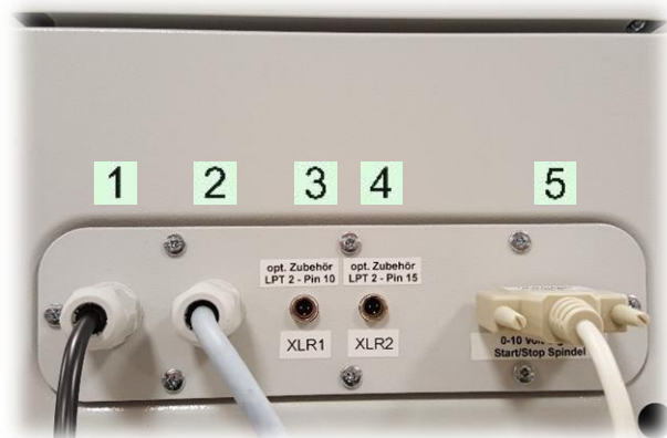
Fig.2: Control cabinet connections
